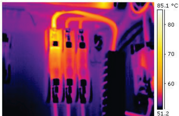
6.2. att. Termogramma elektro sadales skapī ( http://www.ohiothermalinspection.com/ )
